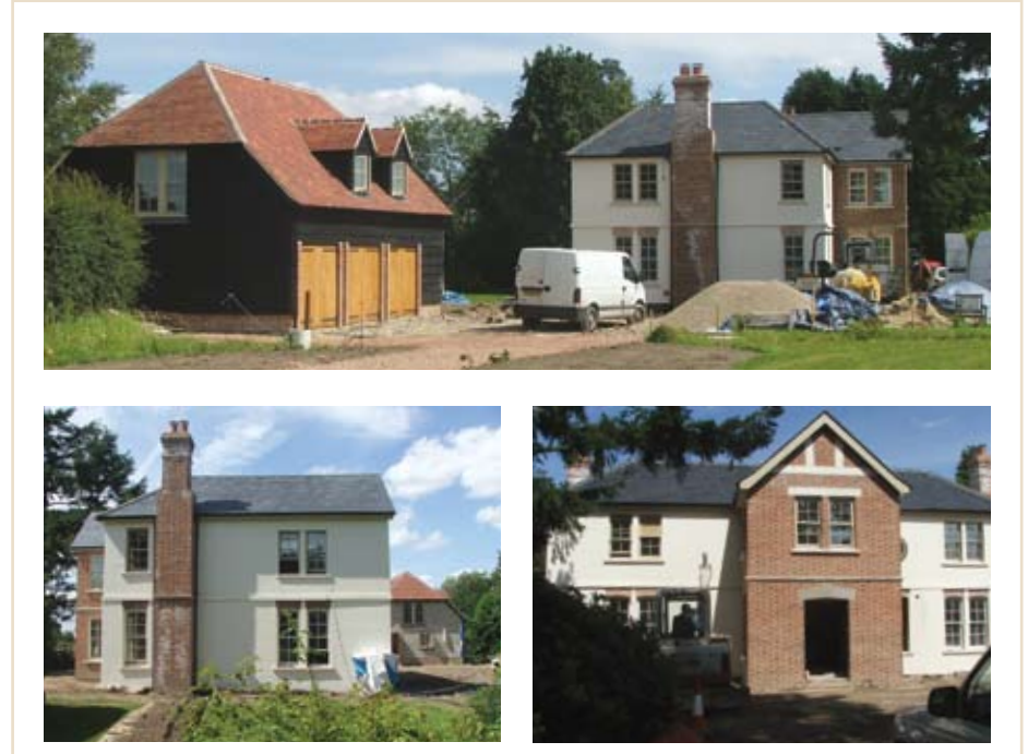
A current project where we were instructed to design and project manage a run down property into something quite spectacular
